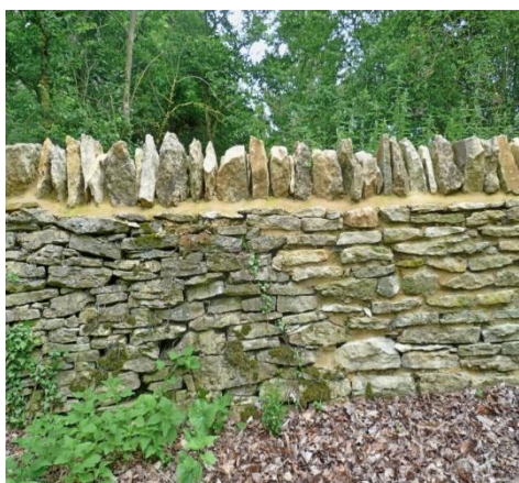
Unmortared v's repaired mortared wall
