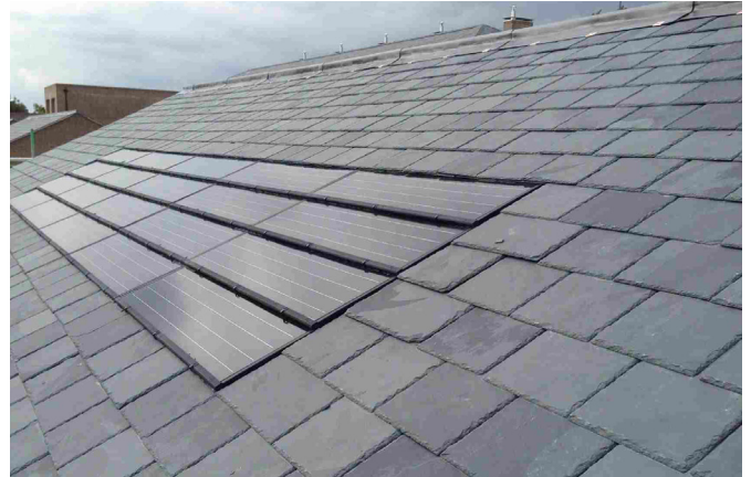
Two examples of a solar panels fitted flush within a natural slate roof (not retrofitted).
