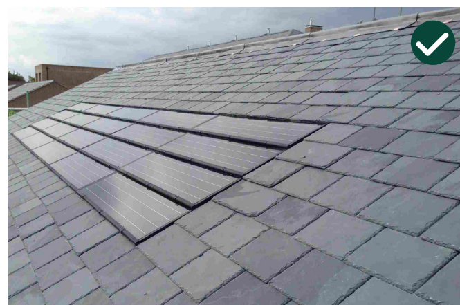
Two examples of a solar panels fitted flush within a natural slate roof (not retrofitted).
